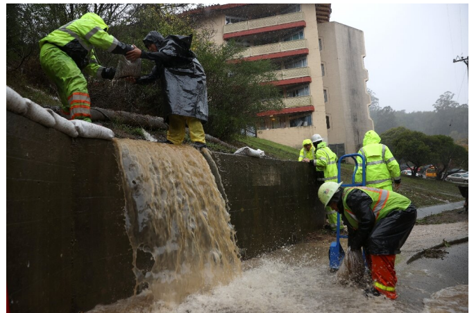
Workers try to divert water into drains in Marin City, California.
