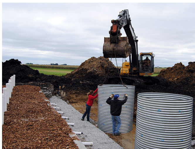
Natasha Hoover (left) and contractors (Con-Struct Inc) install the culverts to be used as sampling wells. Credit: Michelle Soupir
