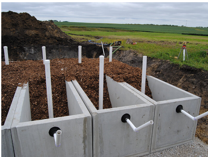
Concrete linings are partially filled with woodchips during installation and monitoring wells are visible. Credit: Michelle Soupir
