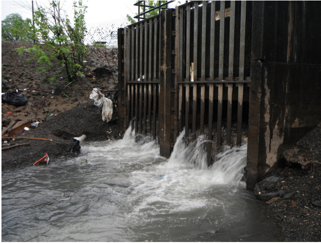
A combined sewer overflow outfall. Credit: U.S. Environmental Protection Agency
