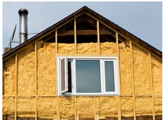
Insulating foam is injected between walls to prevent heat escaping from the home, reducing energy use. Credit: Pi-Lens/Shutterstock
