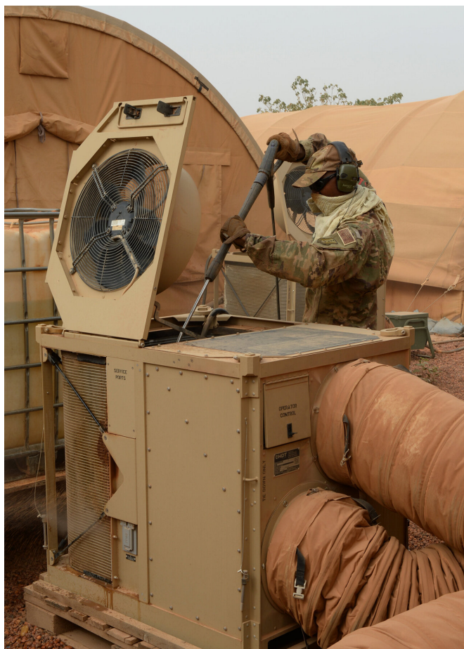
A heating, ventilation and air-conditioning (HVAC) unit gets a cleaning at an Air Force base in Nigeria. Credit: Jimmie Pike/US Air Force
