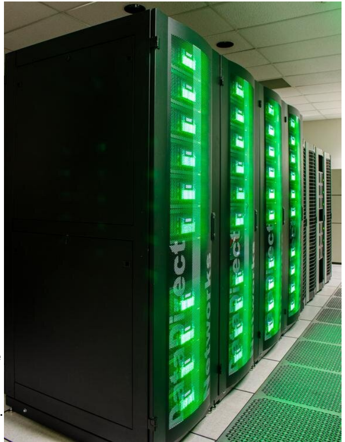
Ranch upgraded to the DDN SFA14K DCR block storage system, supplied by DataDirect Networks, which provides 30 petabytes of spinning disk cache. Credit: TACC
