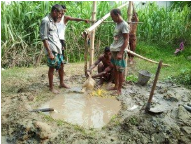
A well installation in Bangladesh. Credit: Rajib Mozumder
