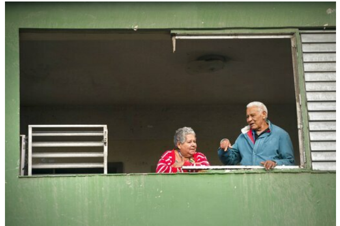
People talk behind a home's window that was destroyed by a tornado in Havana, Cuba, Monday, Jan. 28, 2019. A tornado and pounding rains smashed into the eastern part of Cuba's capital overnight, toppling trees, bending power poles and flinging shards of metal roofing through the air as the storm cut a path of destruction across eastern Havana. (AP Photo/Ramon Espinosa)
