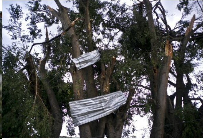
Zinc plates from the roofs of homes are wrapped around a tree after a tornado in Havana, Cuba, Monday, Jan. 28, 2019. A tornado and pounding rains smashed into the eastern part of Cuba's capital overnight, toppling trees, bending power poles and flinging shards of metal roofing through the air as the storm cut a path of destruction across eastern Havana. (AP Photo/Ramon Espinosa)
