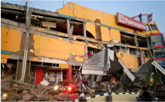
Indonesia's disaster agency released a picture showing a collapsed shopping mall in Palu, Central Sulawesi
