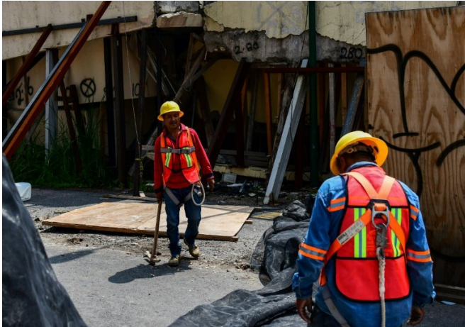
Workers prepare to demolish Enrique Rebsamen elementary school in Mexico city, on August 20, 2018. The school collapsed during the earthquake on September 19 2018, killing 19 children and seven adults
