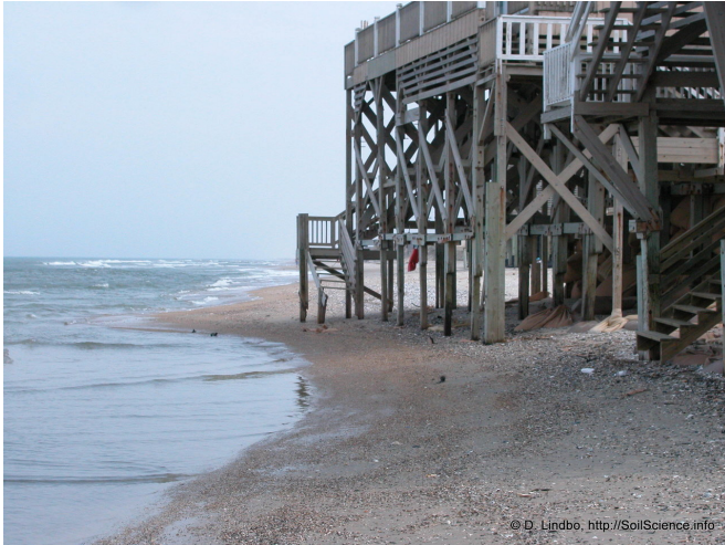
Beach erosion in Nags Head, North Carolina, photographed May 15, 2005. Credit: Soil Science , CC BY
