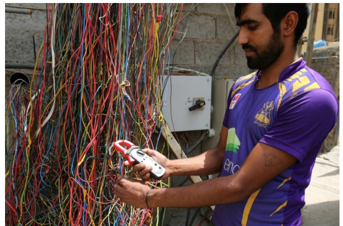
A technician checks wires from a generator supplying homes with electricity in Baghdad on July 26, 2018
