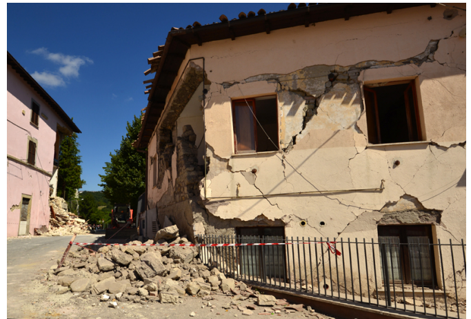
A damaged building at Accumoli by the Amatrice earthquake (August 24, 2016). Credit: Marco Anzidei
