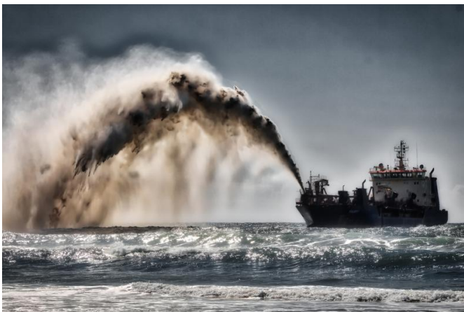
Dredger pumping sand and water to shore for beach renourishment, Mermaid Beach, Gold Coast, Australia, Aug. 20, 2017. Credit: Steve Austin, CC BY-SA
