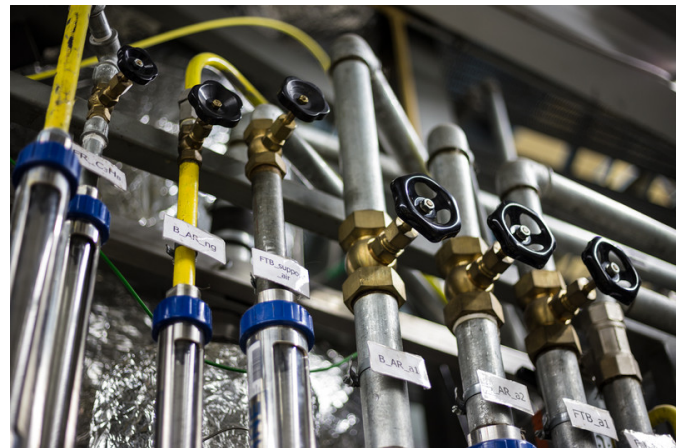
CLC-facility at TU Wien. Credit: Vienna University of Technology
