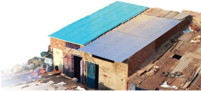
The finished ModRoof material is installed on a home in Gomtipur, an area in the city of Ahmedabad. Credit: ReMaterials
