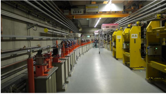
The beamline to connect the FLASHForward experiment to the FLASH accelerator (on the left) is under construction. Credit: Helmholtz Association of German Research Centres
