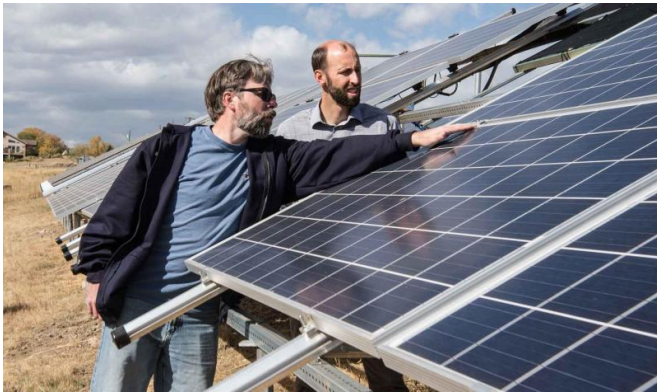
NREL engineers Bill Sekulic (left) and Chris Deline look at the new PV array just north of the NREL parking garage. The new array extends the testing capacity for solar modules at NREL. Credit: Dennis Schroeder
