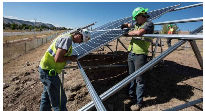
Workers install PV modules just north of the NREL parking garage. Modules in the first row are part of a small demonstration project for the PV industry to help obtain initial performance validation. The PV modules in the other rows are part of a new Energy Department program called PV Lifetime. The intent is to study, with high accuracy, the initial degradation of PV modules, and to make all of the data publicly available. Credit: Dennis Schroeder
