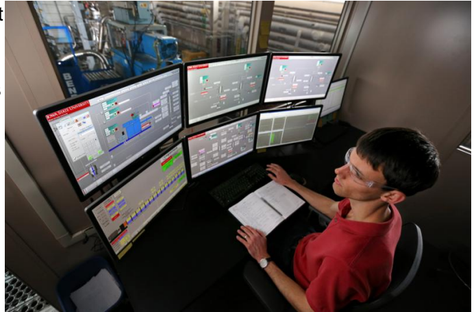
Andrew Friend works the control system of the solvent liquefaction pilot plant. Credit: Iowa State University
