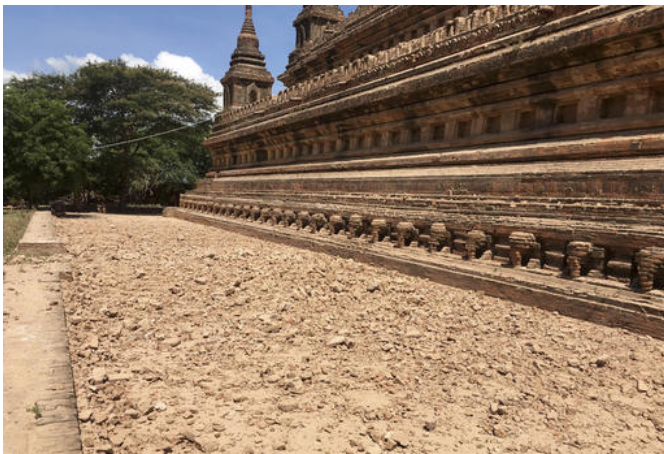
Rubble lies at the base of a temple that was damaged by a strong earthquake in Bagan, Myanmar, Thursday, Aug. 25, 2016. Rescue workers surveyed the damage Thursday after a powerful earthquake shook Myanmar Wednesday, damaging 185 ancient Buddhist pagodas in the former capital of Bagan, a major tourist site. (AP Photo/Min Kyi Thein)
