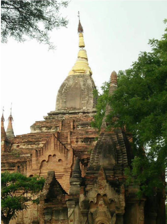
This photo provided by Soe Thura Lwin shows a damaged temple in Bagan, Myanmar, on Wednesday, Aug. 24, 2016. A powerful earthquake measuring a magnitude 6.8 shook central Myanmar on Wednesday, damaging scores of ancient Buddhist pagodas in Bagan, a major tourist attraction, officials said. (Soe Thura Lwin via AP)
