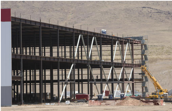
Construction continues on the new Tesla Gigafactory during a media tour Tuesday, July 26, 2016, in Sparks, Nev. It's Tesla Motors' biggest bet yet: A massive, $5 billion factory in the Nevada desert that could almost double the world's production of lithium-ion batteries by 2018. (AP Photo/Rich Pedroncelli)
