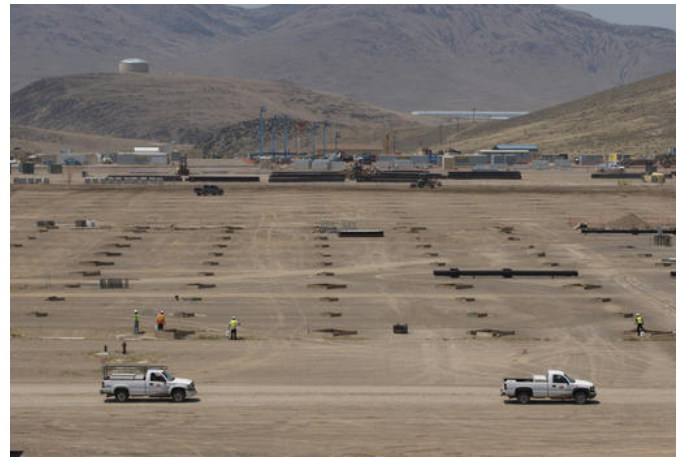
Construction continues at Section F of the new Tesla Gigafactory during a media tour Tuesday, July 26, 2016, in Sparks, Nev. It's Tesla Motors' biggest bet yet: A massive, $5 billion factory in the Nevada desert that could almost double the world's production of lithium-ion batteries by 2018. (AP Photo/Rich Pedroncelli)
