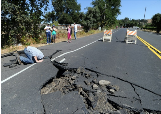
Local resident inspects a buckled highway outside of Napa, California, after earthquake struck the area in the early hours of August 24, 2014
