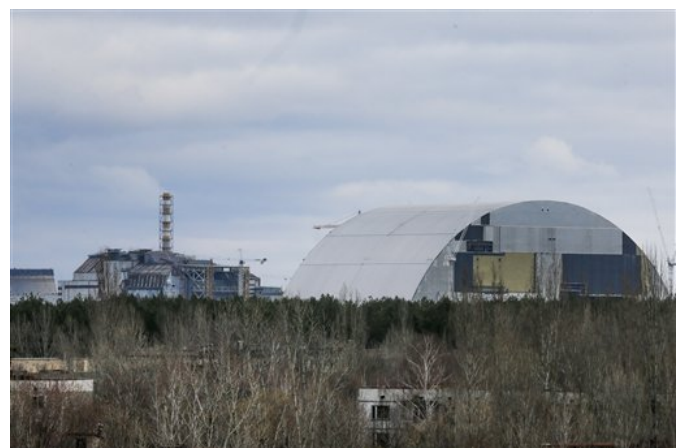
In this photo taken on Wednesday, March 23, 2016, A chimney over the destroyed reactor at the Chernobyl nuclear power plant, background left, and a gigantic steel-arch under construction to cover the remnants of the exploded reactor, in the town of Prypyat close to Chernobyl, Ukraine. Abandoned houses in the
