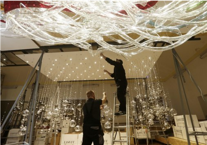
In this picture taken on Thursday, Feb. 18, 2016, workers adjust a piece of installation designed for Lasvit glass maker at a warehouse in Pysk, Czech Republic. Lasvit founders' goal was to combine the traditional glass blowing techniques that date to the 12th century in the Czech lands known as Bohemia with the latest technology and work of top contemporary designers, both domestic and international. (AP Photo/Petr David Josek)
