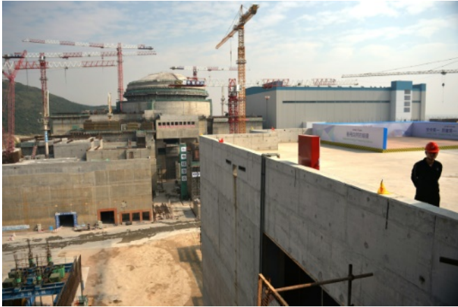
Construction under way on the Taishan Nuclear Power Station outside Taishan City in Guangdong province on December 8, 2013
