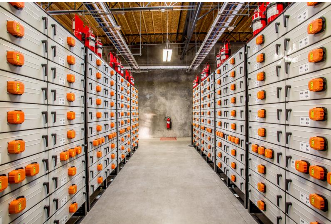
Portland General Electric installed a 5-megawatt, lithium-ion battery in Salem, Oregon, as part of the Pacific Northwest Smart Grid Demonstration Project. Credit: Portland General Electric
