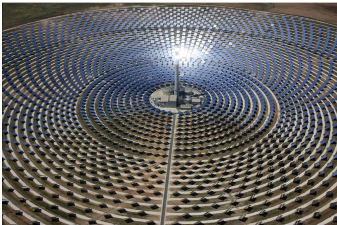
The Gemasolar solar power plant, situated near Seville in Spain. Credit: Torresol Energy
