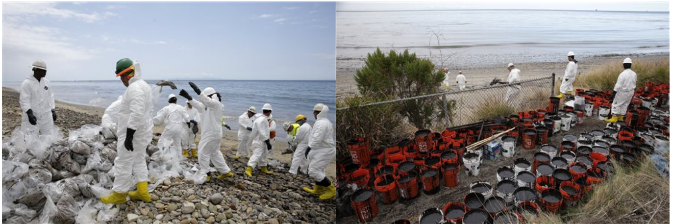
Clean up workers gather oil-contaminated sand bags at Refugio State Beach, north of Goleta, Calif., Thursday, May 21, 2015. More than 7,700 gallons of oil has been raked, skimmed and vacuumed from a spill that stretched across 9 miles of California coast, just a fraction of the oil escaped from a broken pipeline, officials said. (AP Photo/Jae C. Hong)
