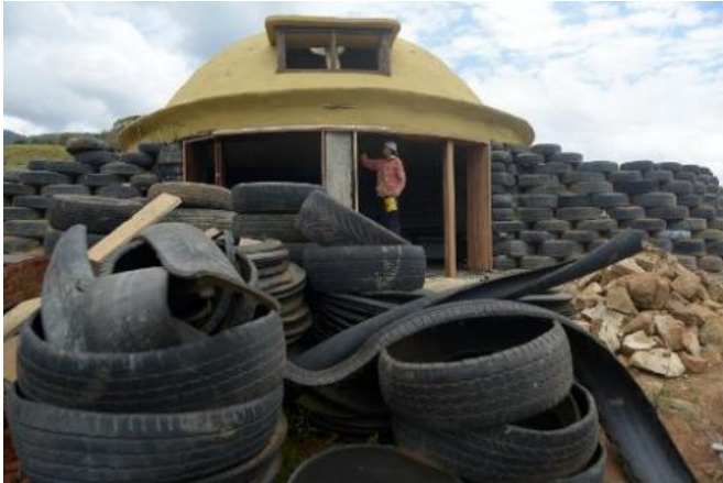
A man works building a house with tires in Choachi, Colombia on March 16, 2015
