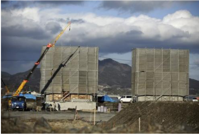
In this March 5, 2015 photo, workers build sea walls in Rikuzentakata, Iwate Prefecture, northeastern Japan. Four years after a towering tsunami ravaged much of Japan's northeastern coast, efforts to fend off future disasters are focusing on a nearly 400-kilometer (250 mile) chain of cement sea walls, at places nearly five stories high. (AP Photo/Eugene Hoshiko)
