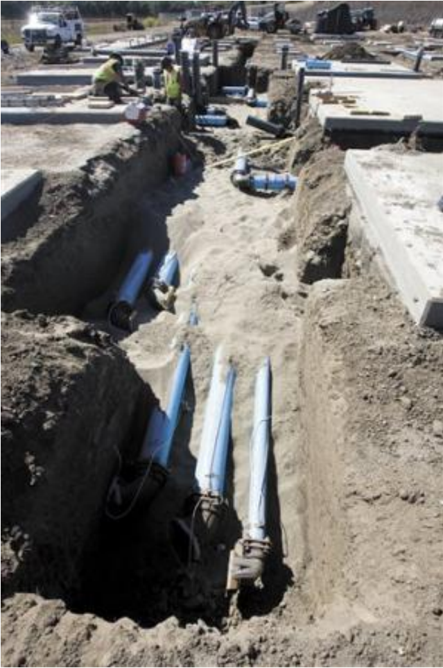
In an Oct. 2, 2014 photo, the Cambria Community Services District works on a desalination plant, in Cambria, Calif. Drought has lowered water levels in the district. Water for the desalination plant under construction will enter the plant in the foreground and go through a series of processes. Cambria is opening the plant under a state drought-emergency declaration, using a novel mix of brackish estuary water, fresh water, and more than a bit of recycled sewage wastewater. (AP Photo/The Tribune (of San Luis Obispo), David Middlecamp)
