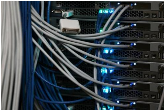
Network cables in a server room seen on November 10, 2014 in New York
