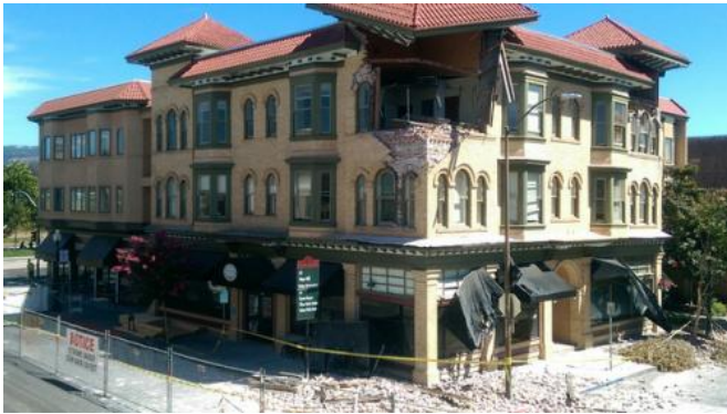
Napa's landmark Alexandria Hotel & Annex, built in 1910, was badly damaged by the 6.0 earthquake on Aug. 24 – despite seismic retrofitting years ago. Credit: Wikimedia Commons user Cullen328
