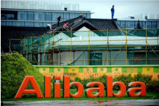
Workers renovate a building at the Alibaba head office in Hangzhou, east China's Zhejiang province on September 15, 2014
