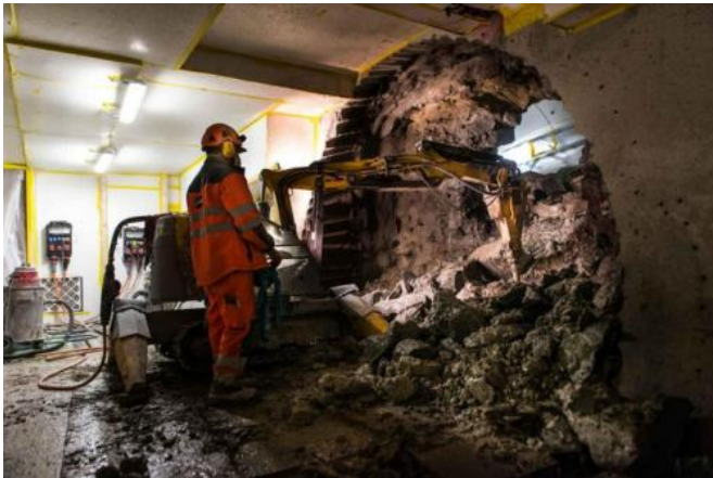
Construction work is already underway at CERN for the AWAKE project. Credit: Maximilien Brice/CERN
