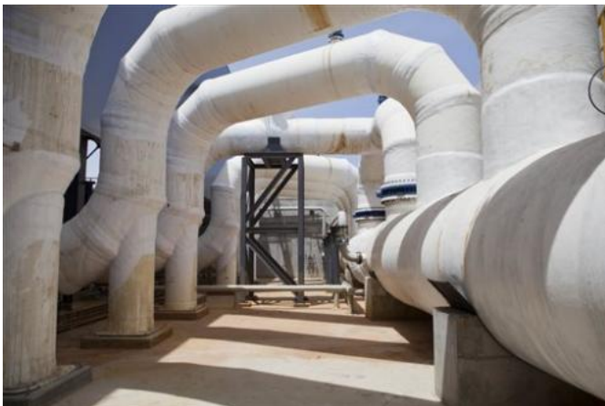
This Sunday, May 4, 2014 photo shows Sorek desalination plant in Rishon Letzion, Israel. Israel's aggressive desalination program that has transformed this perennially parched country into perhaps the most well-hydrated country in the region. (AP Photo/Dan Balilty)
