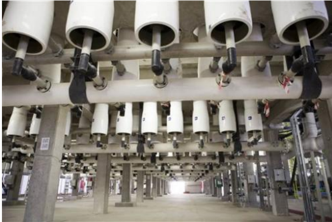
This Sunday, May 4, 2014 photo, shows Sorek desalination plant in Rishon Letzion, Israel. Israel's aggressive desalination program that has transformed this perennially parched country into perhaps the most well-hydrated country in the region.. (AP Photo/Dan Balilty)
