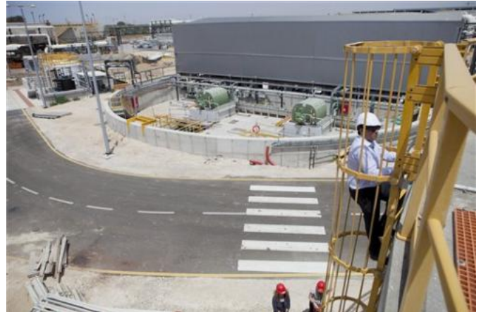
This Sunday, May 4, 2014 photo shows the Sorek desalination plant in Rishon Letzion, Israel. Israel's aggressive desalination program that has transformed this perennially parched country into perhaps the most well-hydrated country in the region. (AP Photo/Dan Balilty)
