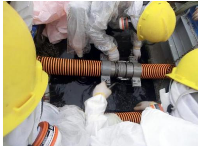
Image provided by TEPCO on October 9, 2013 shows workers checking pipe joints at a decontamination facility at the Fukushima nuclear plant at Okuma town
