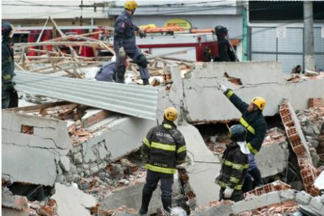
Rescuers work amid the rubble of a building in construction that collapsed in Sao Paulo, Brazil, on August 27, 2013.
