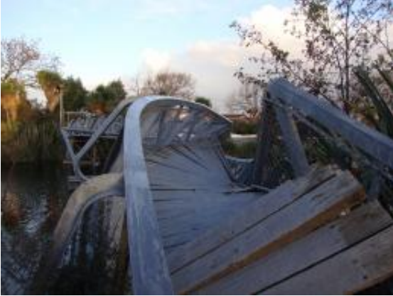
Medway footbridge over the Avon River after the earthquake. Credit: Schwede66
