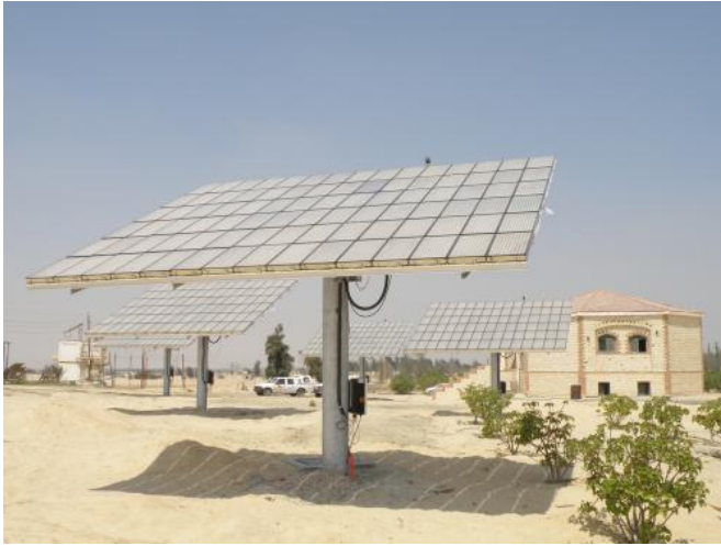
The concentrating photovoltaic modules in Egypt are precisely aligned to the sun. They supply power to irrigate wheat fields. (© Fraunhofer ISE)
