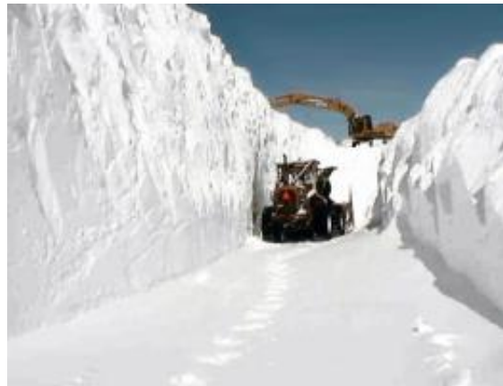
This image of Trans-Labrador Highway, located in Canada's province of Newfoundland and Labrador, shows a heavy excavator bucket and a snow plow clearing snow from the road. Credits: A. Khan, Government of Newfoundland and Labrador
