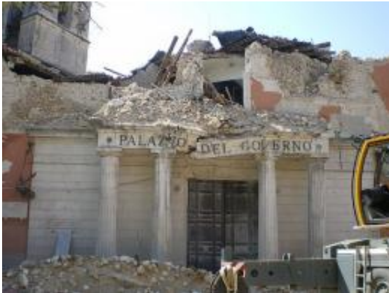
A government's office damaged by the L'Aquila earthquake in 2009. Image credit: Wikimedia Commons.
