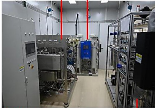
10000 kg/year green ammonia production system
