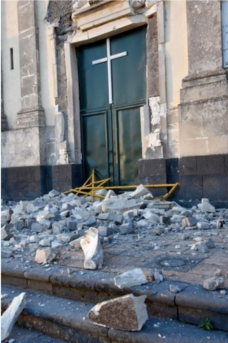
Debris stand in front of the heavily damaged church of Maria Santissima in Fleri, Sicily Italy, Wednesday, Dec. 26, 2018. A quake triggered by Italy's Mount Etna volcano has jolted eastern Sicily, slightly injuring 10 people and prompting frightened Italian villagers to flee their homes. (Orietta Scardino/ANSA Via AP)
