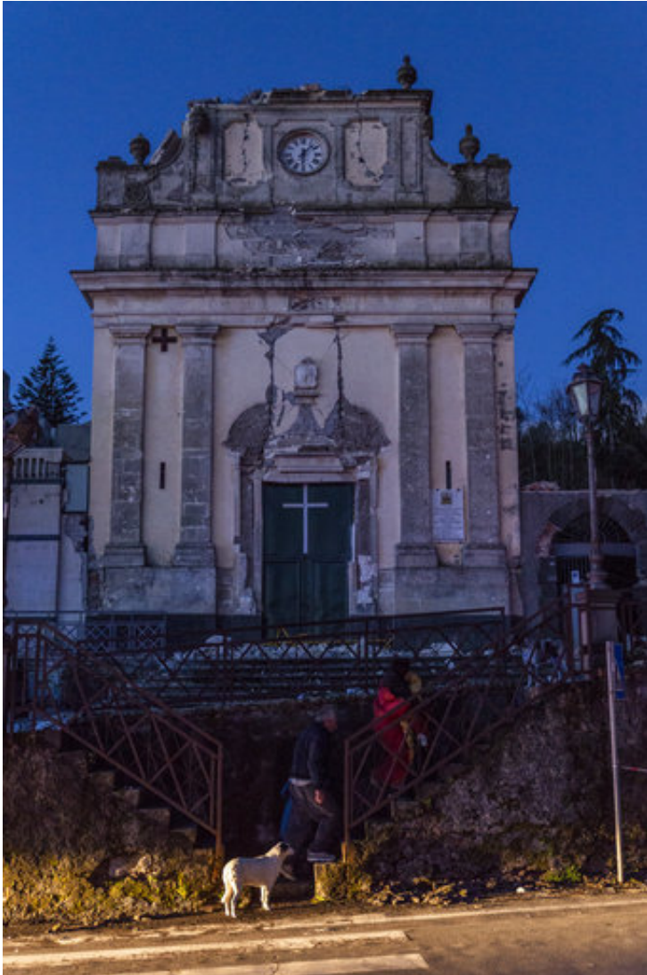
People walk in front of the heavily damaged church of Maria Santissima in Fleri, Sicily Italy, Wednesday, Dec. 26, 2018. A quake triggered by Italy's Mount Etna volcano has jolted eastern Sicily, slightly injuring 10 people and prompting frightened Italian villagers to flee their homes. (AP Photo/Salvatore Allegra)
