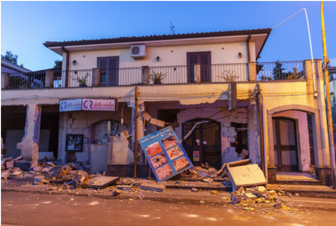
Debris sit on the street in front of an heavily damaged house in Fleri, Sicily Italy, Wednesday, Dec. 26, 2018. A quake triggered by Italy's Mount Etna volcano has jolted eastern Sicily, slightly injuring 10 people and prompting frightened Italian villagers to flee their homes. (AP Photo/Salvatore Allegra)
