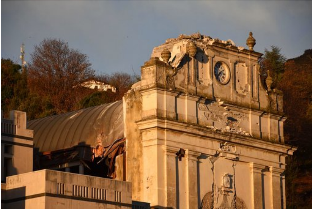
A view of the heavily damaged church of Maria Santissima in Fleri, Sicily Italy, Wednesday, Dec. 26, 2018. A quake triggered by Italy's Mount Etna volcano has jolted eastern Sicily, slightly injuring 10 people and prompting frightened Italian villagers to flee their homes. (Orietta Scardino/ANSA Via AP)
