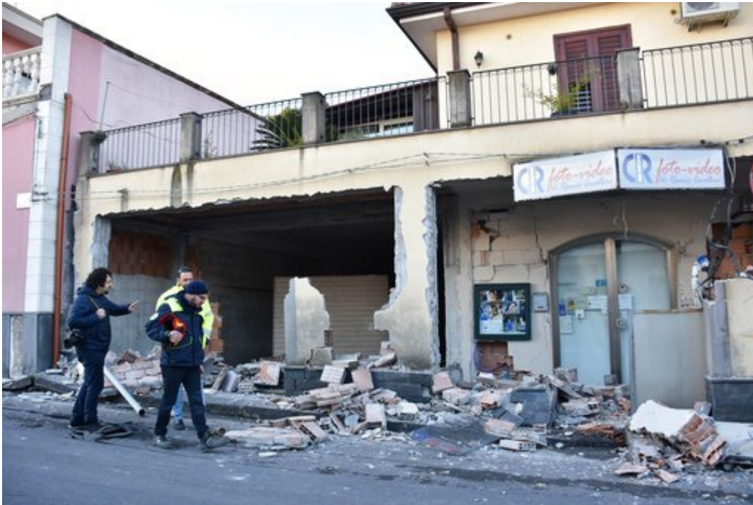
People walk past an heavily damaged house in Fleri, Sicily Italy, Wednesday, Dec. 26, 2018. A quake triggered by Italy's Mount Etna volcano has jolted eastern Sicily, slightly injuring 10 people and prompting frightened Italian villagers to flee their homes. (Orietta Scardino/ANSA Via AP)
