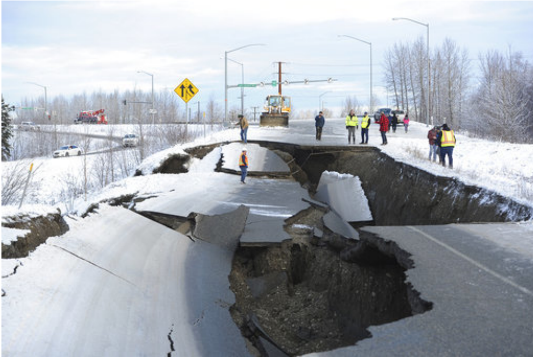
Workers inspect an off-ramp that collapsed during a morning earthquake, Friday, Nov. 30, 2018, in Anchorage, Alaska. (AP Photo/Mike Dinneen)
