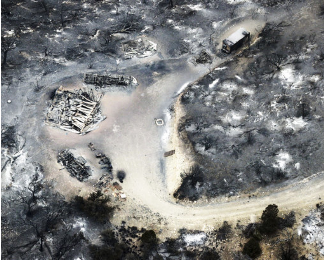
This photo shows burned structures caused by a wildfire near Duchesne, Utah, Thursday, July 5, 2018. (Ravell Call/The Deseret News via AP)
