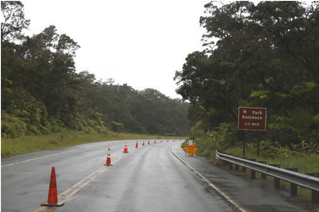
Cones and signs warn of cracks in the road caused by earthquakes near the entrance to Hawaii Volcanoes National Park, Thursday, May 17, 2018, near Volcano, Hawaii. (AP Photo/Caleb Jones)
