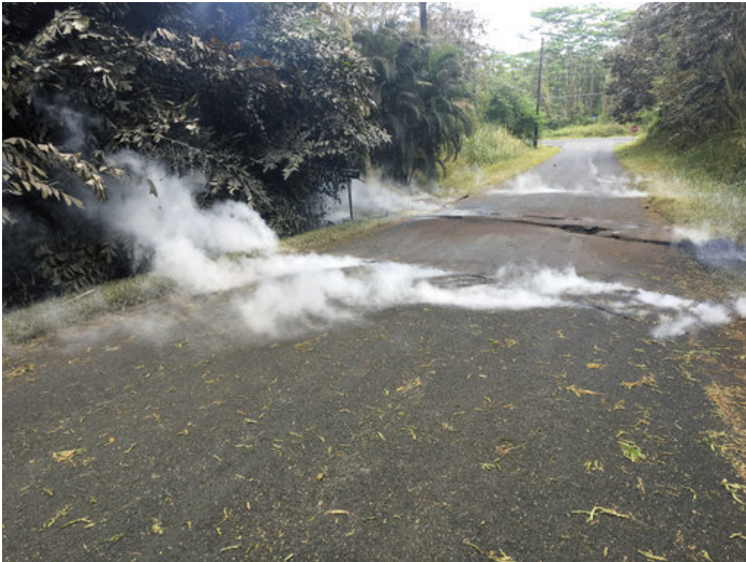
Fumes come out of cracks on the asphalt road near the Leilani Estates in Pahoa,
