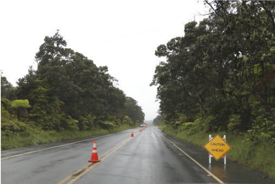
Cones and signs warn of cracks in the road near the entrance to Hawaii Volcanoes National Park, Thursday, May 17, 2018, near Volcano, Hawaii. (AP Photo/Caleb Jones)
