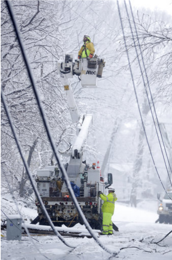
Utility workers use a bucket truck to work on downed power lines along Mountainside Drive ahead of a winter storm, Wednesday, March 7, 2018, in Morristown, N.J. Residents are gearing up for a second storm after last week's weather downed trees and power lines. (AP Photo/Julio Cortez)
