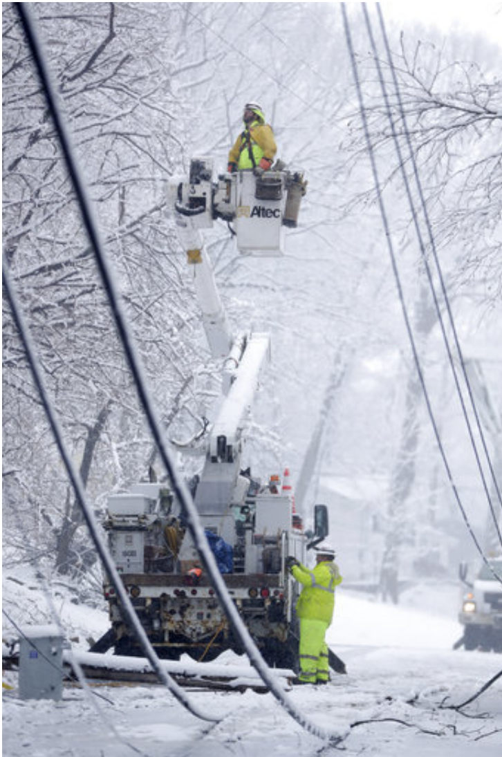
Utility workers use a bucket truck to work on downed power lines along Mountainside Drive ahead of a winter storm, Wednesday, March 7, 2018, in Morristown, N.J. Residents are gearing up for a second storm after last week's weather downed trees and power lines. (AP Photo/Julio Cortez)
